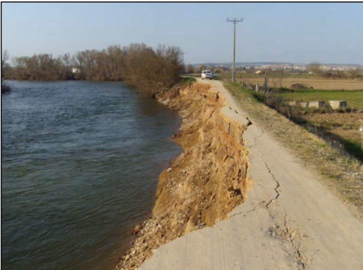
Figure 5. View of a partial failure of a levee caused by the slope erosion in contact with the water flow.
