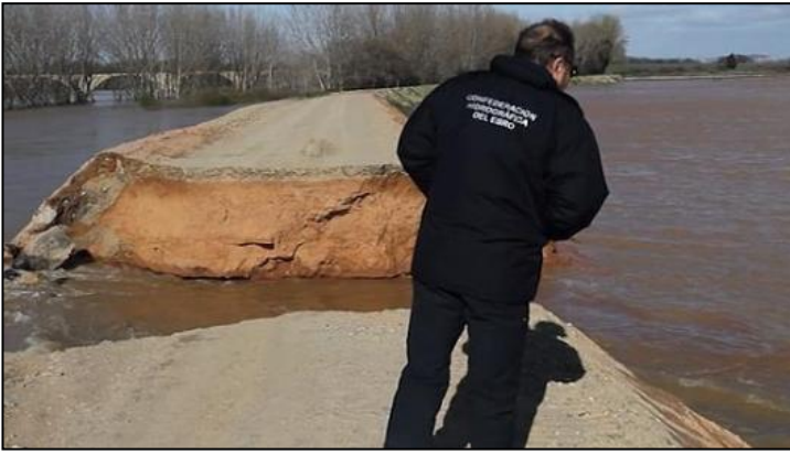
Figure 6. Example of partial failure in a levee due to an inadequate foundation.
