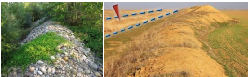
Figure 2. Different types of levee built out of material available in the riverbed: River Curueño and River Valdeginatate (River Douro basin).
