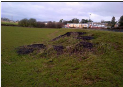
Photograph showing badger damage to a levee – courtesy of Environment Agency
