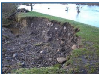
Severe levee erosion along the River Tyne – Dilston Haughs. Image credit: HR Wallingford
