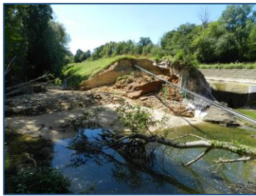
Breach on the right bank of Canal de Briare Photo credit IRSTEA
